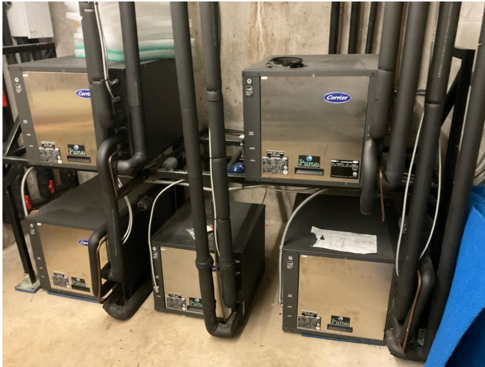
Figure 7: Direct-exchange geothermal temperature control system indoor units at 76 Morison Drive.
