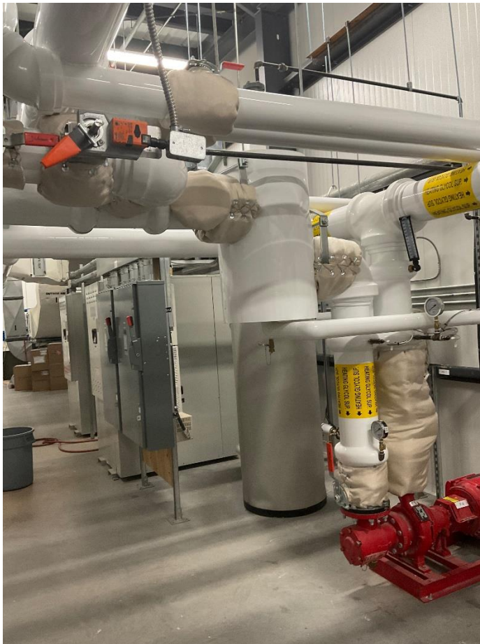
Figure 10: Glycol heating and cooling system operating room at West Hants Sports Complex.
