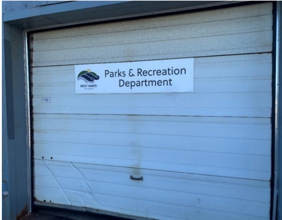
Figure 5: Parks and Recreation workshop exterior door received an energy efficiency rating of 0% and should be heavily considered for upgrade. Significant outside air infiltration, rust along edges, and physical damage were observed.
