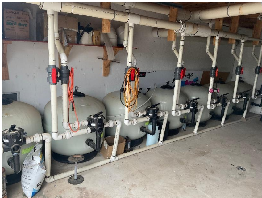
Figure 9: Electric pumps at 306 Stannus St.
