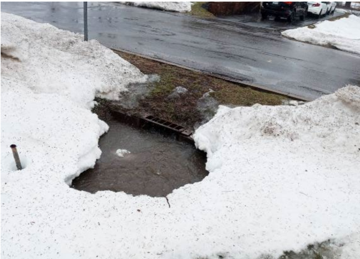
Figure 20 Culvert backed up within the system causing year-round flood risk and property damage
