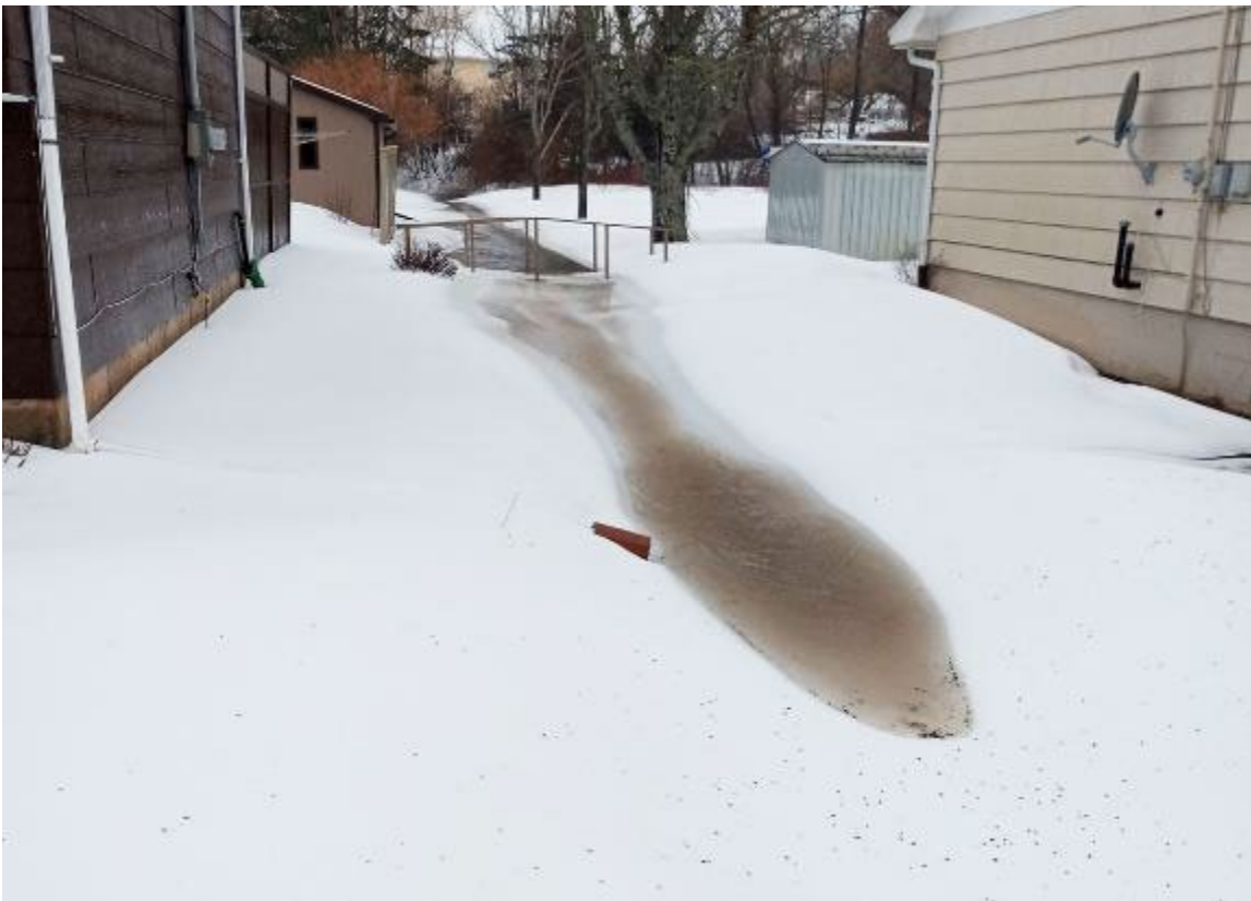
Figure 18 Winter flooding and frozen ditching backing up at Tremain culvert
