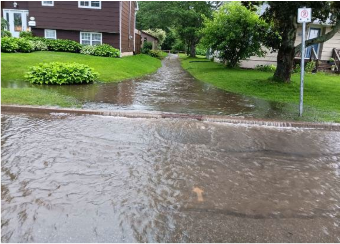
Figure 9 Culvert fully backed up with flows running fully over curb and street
