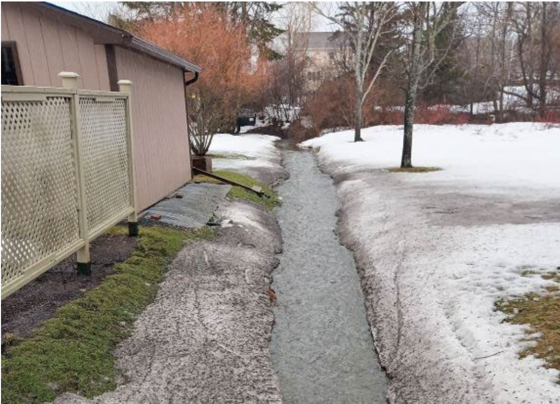
Figure 19 Winter flooding within ditching due to backed up culvert
