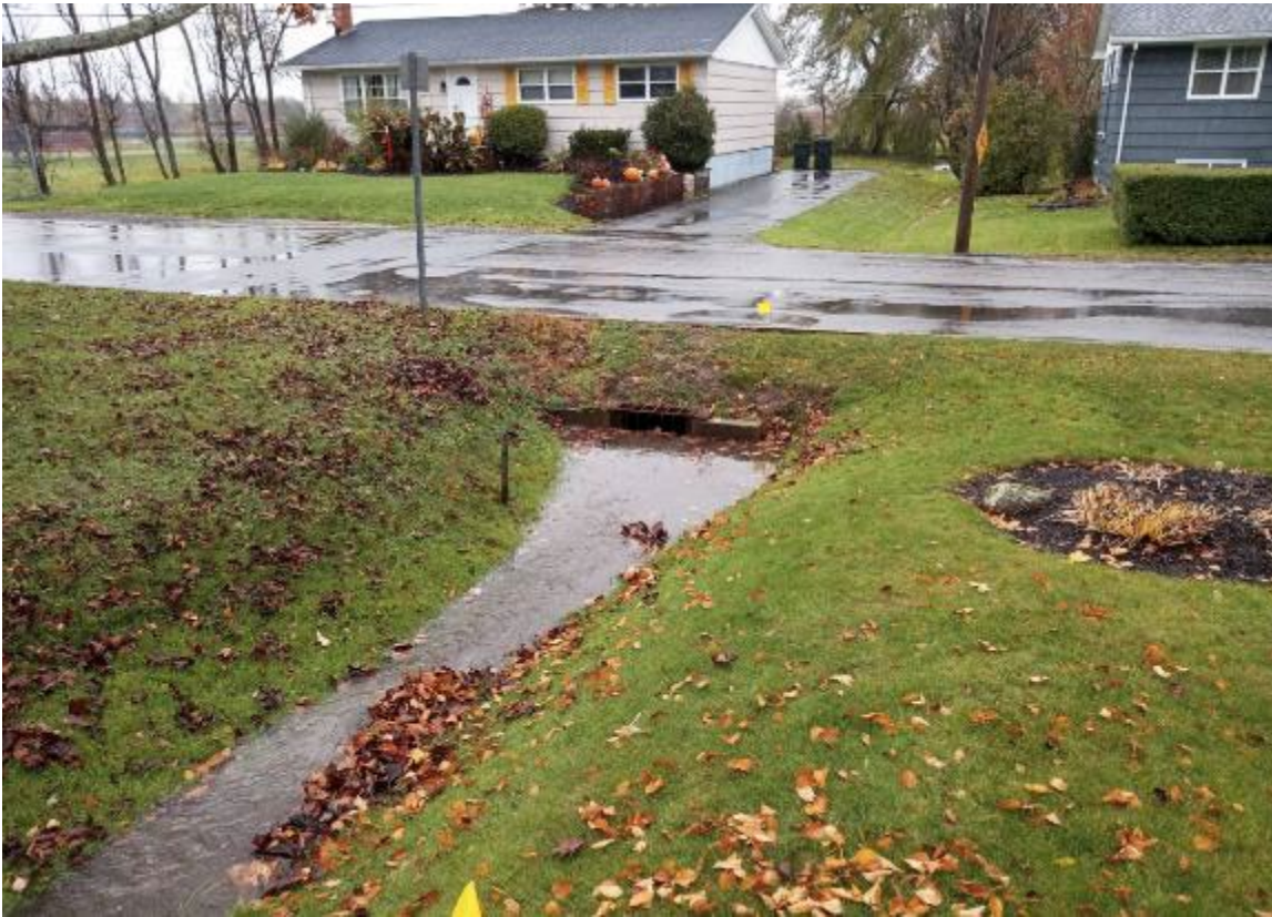
Figure 3 Flood water rising to top of ditch and culvert
