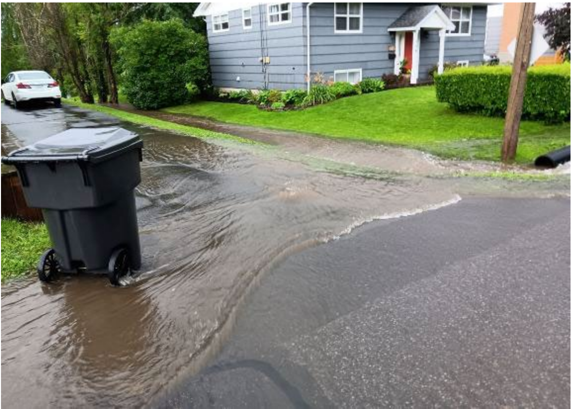
Figure 10 Flood water from across the street and open -incomplete culvert at right driveway
