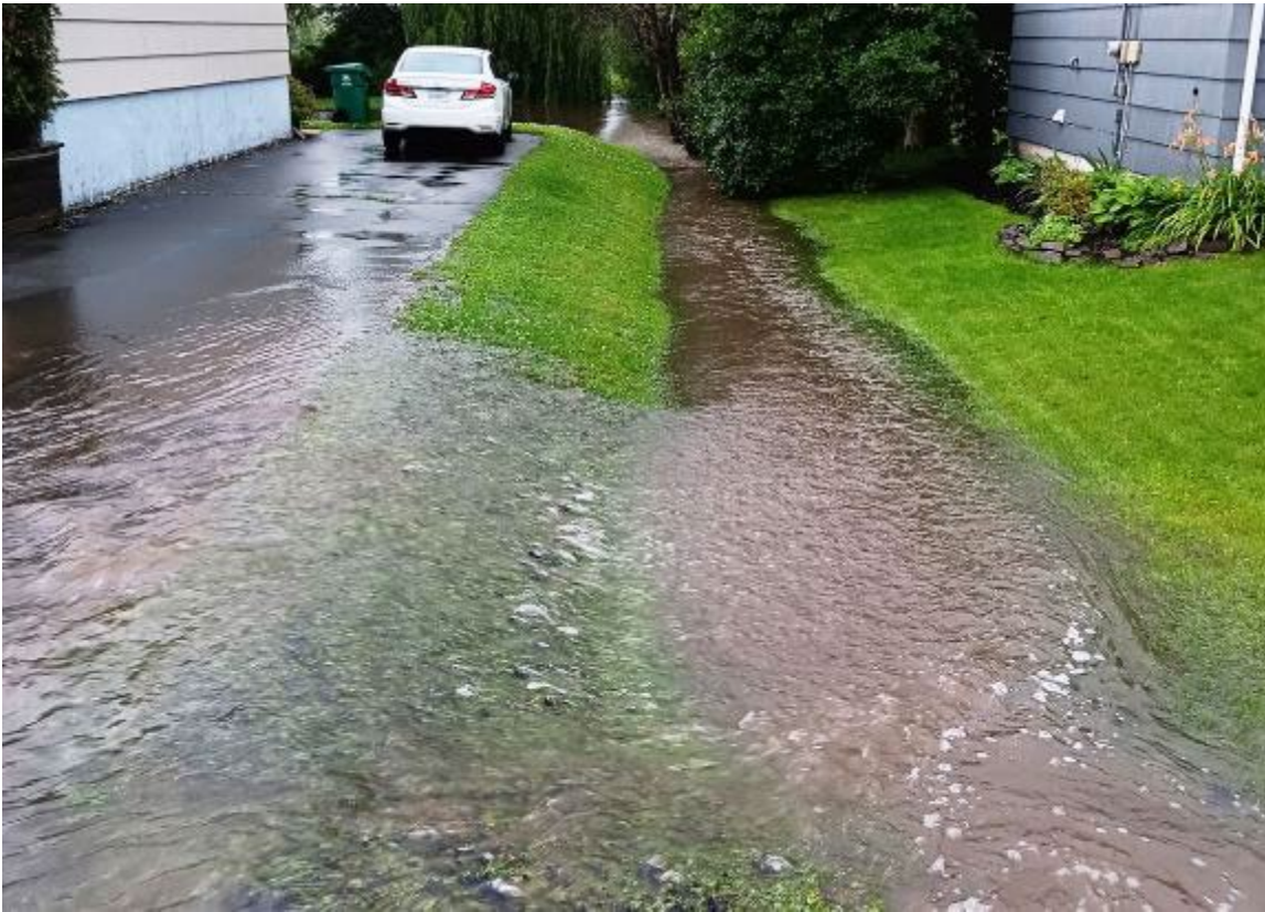
Figure 11 Floodwater from street & incomplete / open culvert between properties across the street.
