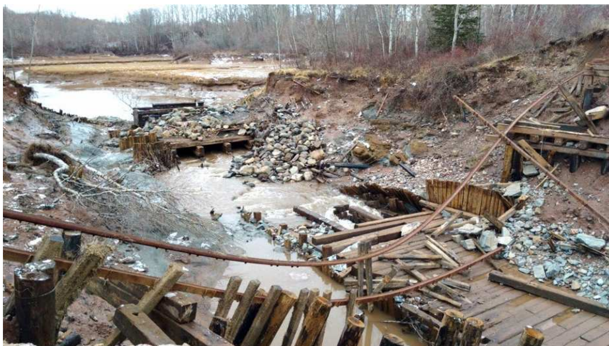
Figure 3: Mouth of HWR post-failure with aboiteau, construction material and rail line remaining within the crossing (breach) location. Photograph by CBWES Inc 2018.
