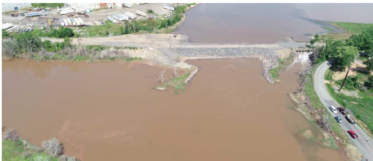
Figure 5: Causeway at high spring tide (July 7, 2020), tidal ingress occurring through main culvert, evidenced by upwelling, and through the overflow culverts.. Drone Imagery by CBWES 2020.
