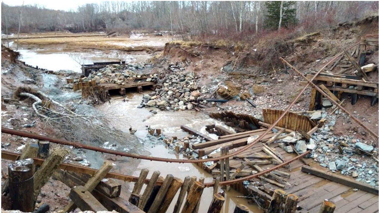
Figure 3 Part of the aboiteau, construction material and rail line remain within the crossing (breach) location and continue to negatively impact the hydrology. Note – the rail lines visible in this picture from February 2018 have since been removed for safety reasons. Photograph by CBWES Inc.
