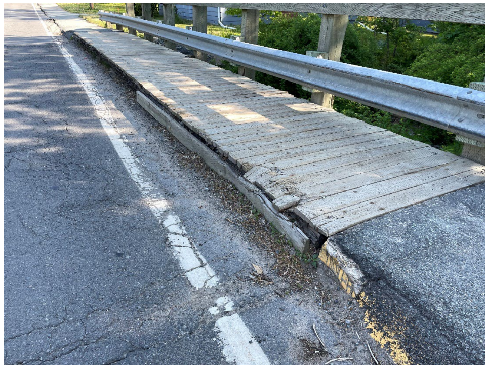
Willow Bridge Sidewalk Condition (width insufficient for safe snow clearing operations)
