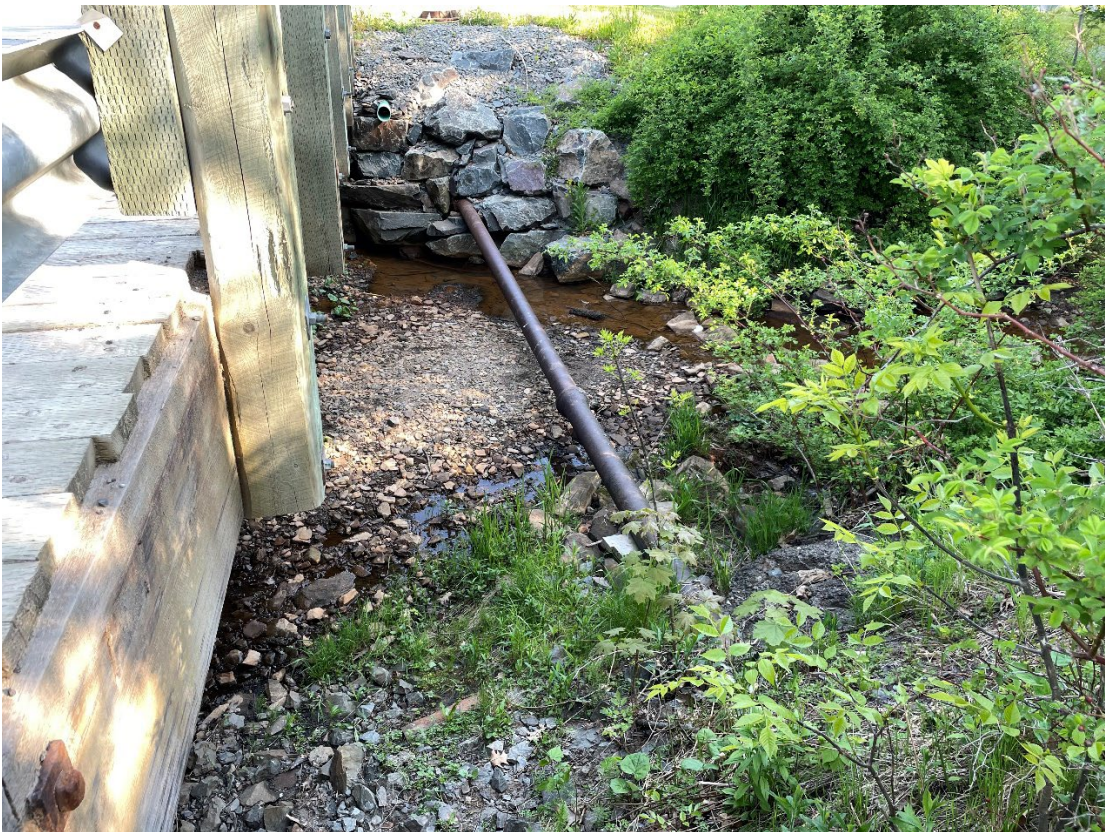
Exposed Sanitary Sewer Main within Willow Brook (under drought conditions)
