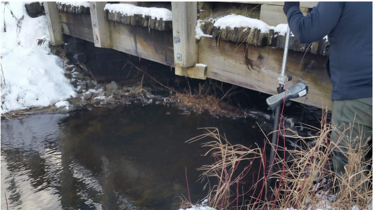
Figure 3-5: Panuke Road Bridge debris buildup – looking downstream from upstream end (November 22, 2018)
