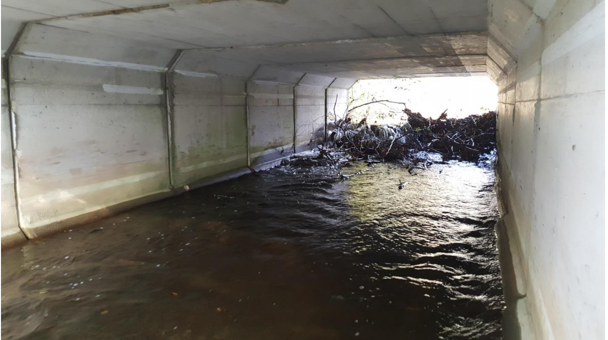
Figure 3-4: WTP access road culvert (1 of 4) debris buildup – looking upstream from downstream end (October 15, 2018)
