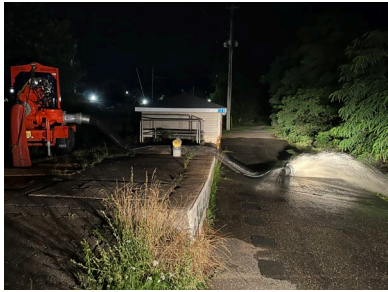
WHRM Pump at waterfront lift station, Windsor, NS
