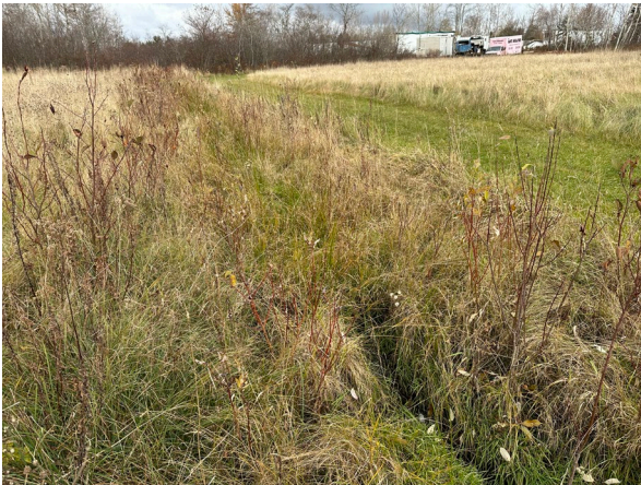
Photo 3: Ditch completely infills and dries approximately 190 m north of Windsor Back Road.
